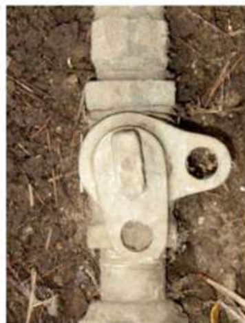
Water meter shutoff at the street and shutoff tool
